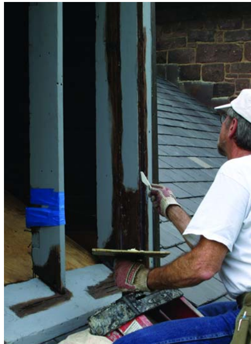
Window sash was removed, repaired, and refinished at Hoffman Painting & Refinishing's shop in Pipersville, PA. Here, Hoffman journeyman wood restorer Mike Orrell is shown at work repairing window frames and sills, which were restored in place at the Cornwall Furnace historic site.
