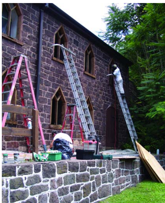
Craftsmen with Hoffman Painting & Refinishing at work during restoration of the windows at the iron furnace. Photos courtesy of Pennsylvania Historical and Museum Commission, Craig A. Benner photographer
